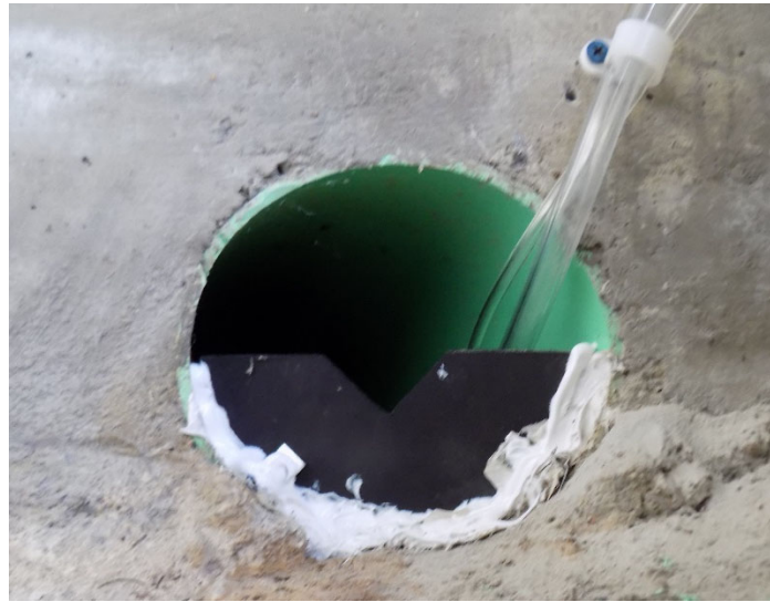
Figure 6-5. V-Notch Weir with Sampler and Bubbler Installation in Underdrain
