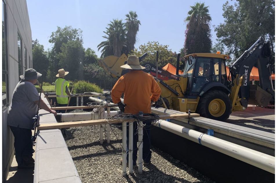
For more than two decades, the SMC has helped rally southern California's stormwater management community around a common vision for BMPs as a solution for protecting the health of the region's waterways. Above, a bioretention BMP under construction at the Riverside County Flood Control and Water Conservation District.
